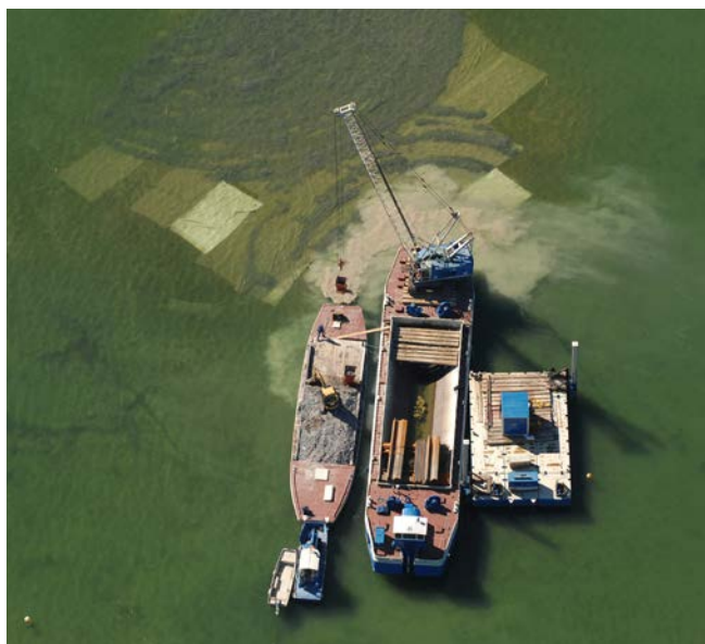
Fig. 1 Covering the archaeological site of Rapperswil-Jona, Technikum, in the shallow water zone of Lake Zurich, Switzerland, with geotextile and gravel. Use of a gravel barge and a crane with jib. © Archaeological Service of the Canton of St. Gallen, Simon Vogt, 2011.
