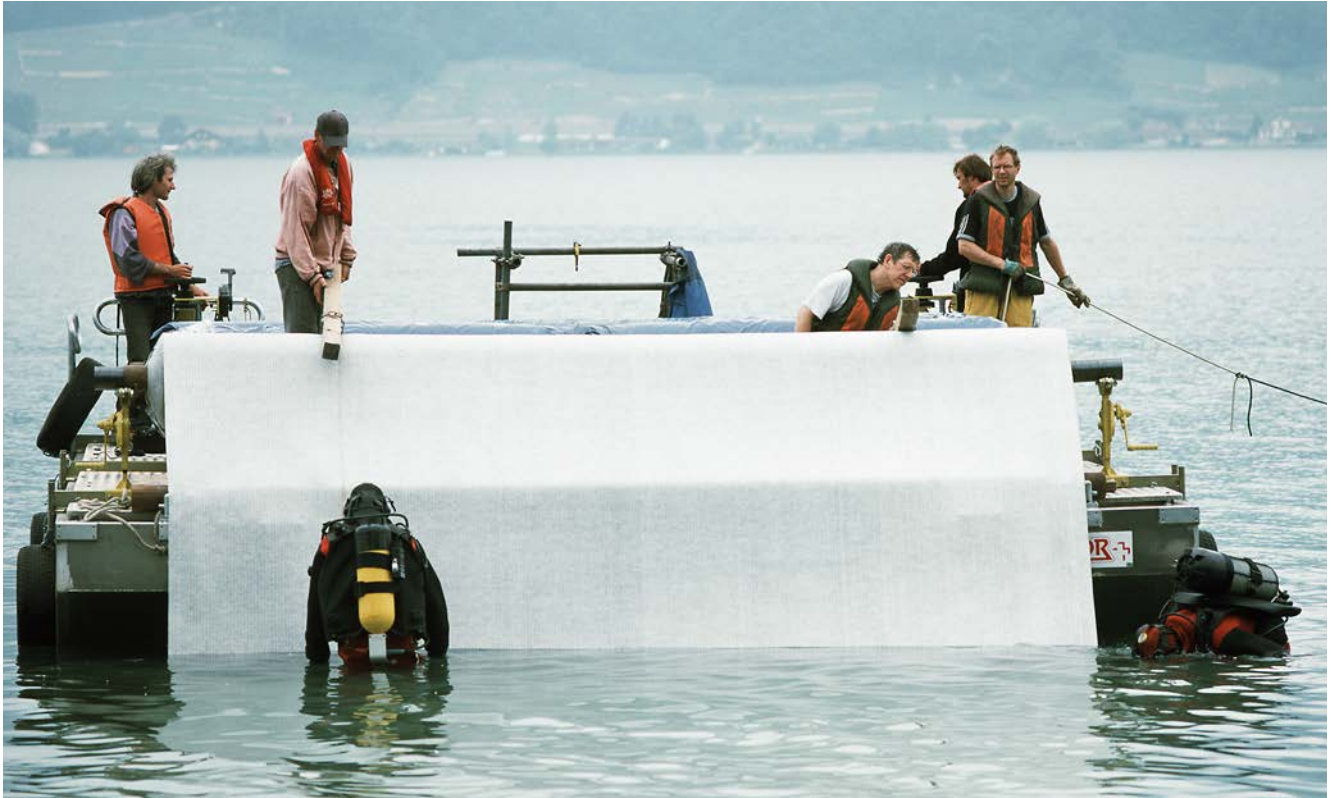
Fig. 4 Spreading of heavy geotextile mats with a sand inlay of 5 m width and 30 m length, which are normally used in road construction. The special ship of the Archaeological Service of the Canton of Bern in an operation on Lake Biel. © Archaeological Service of the Canton of Bern, diving team.
